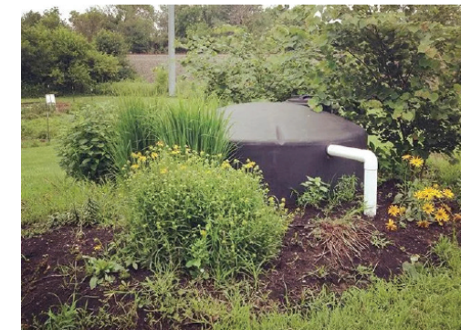
Screened on ground tank
